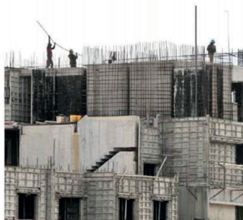
Builders' job flow should accelerate with the roll-out of the MRT3, Penang Light Rail Transit, various flood mitigation projects as well as private-sector projects such as new data centres and semiconductor foundries, analysts observed. — Bernama photo
